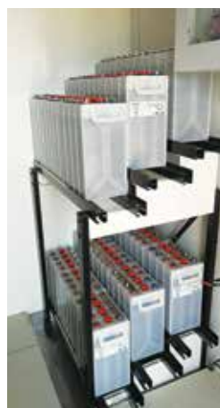
A typical battery system for the Hassi R'Mel pipeline.
